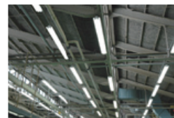
High-frequency inverter lights
